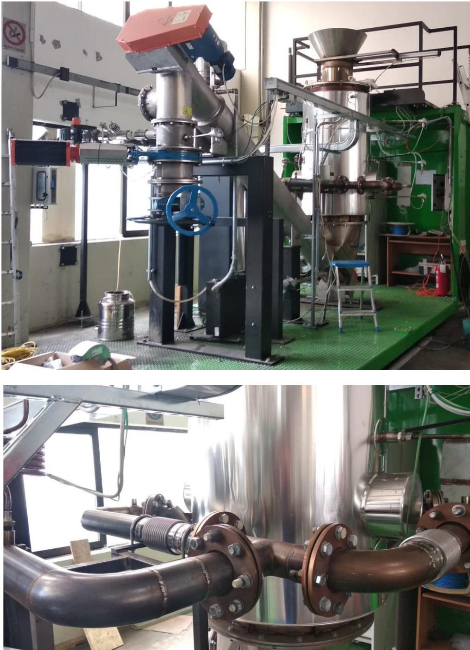
Figure 7: Picture of the new pilot configuration (up) and detail of the vapour extraction section from the reactor (bottom). Insulation removed to show the construction details.
