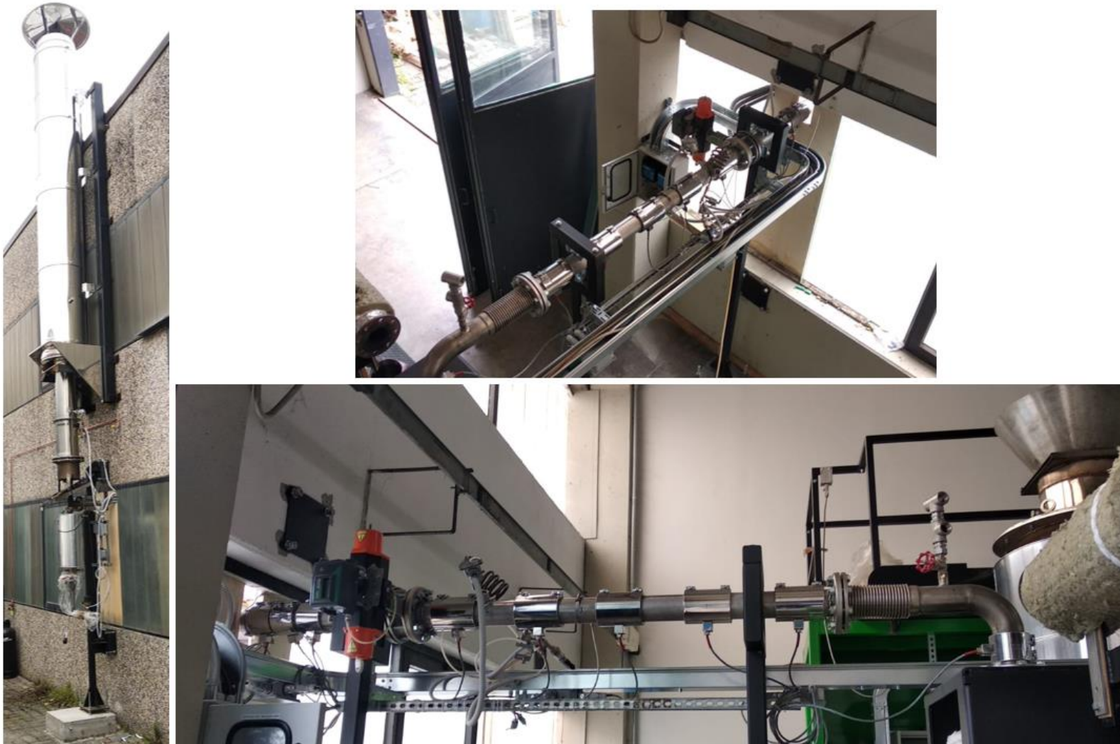
Figure 9: Pictures of the new hot vapours line: new torch (left) and new vapours line with electric heaters (right). Insulation removed to show the construction details.
