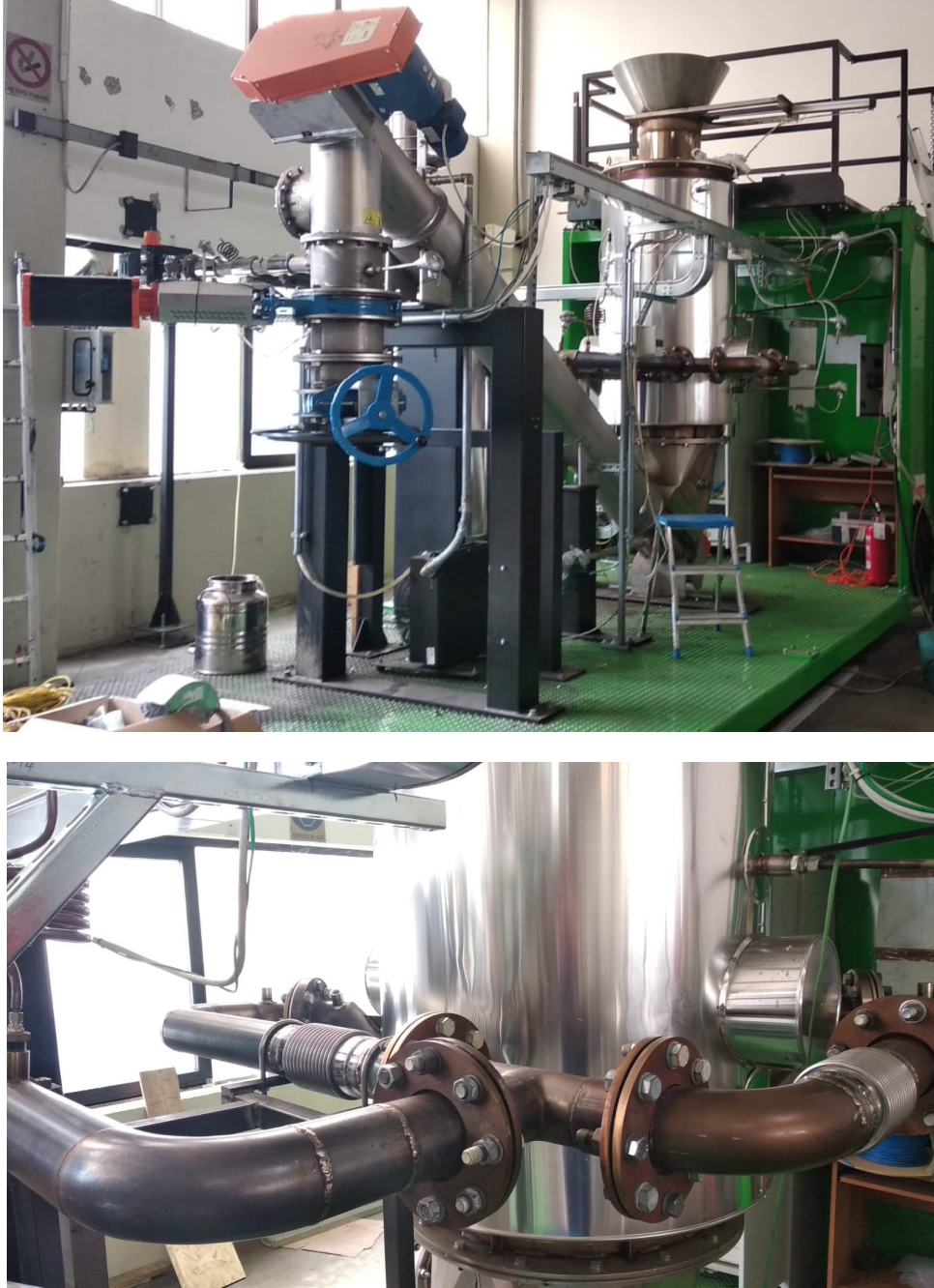
Figure 7: Picture of the new pilot configuration (up) and detail of the vapour extraction section from the reactor (bottom). Insulation removed to show the construction details.
